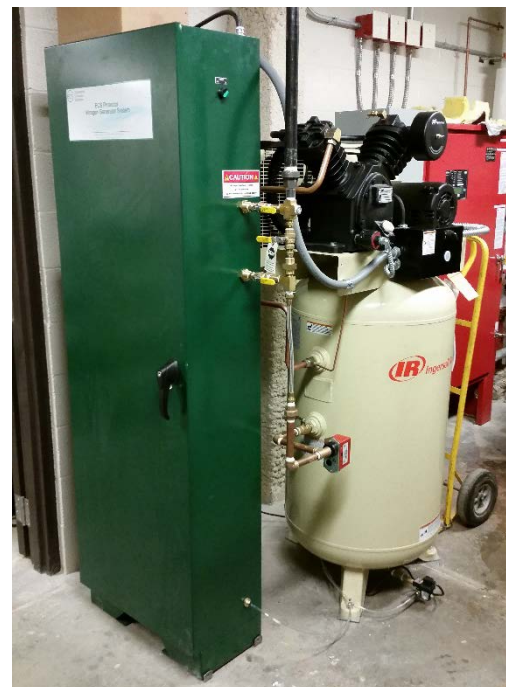
ECS PGEN-40 Nitrogen Generator Installed with Air Compressor
