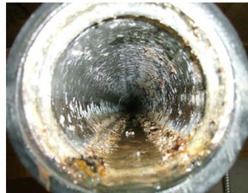
Corroded Galvanized Main with Trapped Water
