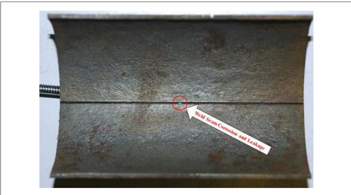
Fig. 12. Preferential grooving corrosion on a pipe weld seam with a .04 in. (1 mm) pinhole leak in a wet pipe system, after removing corrosion products inside an NPS 3 pipe
