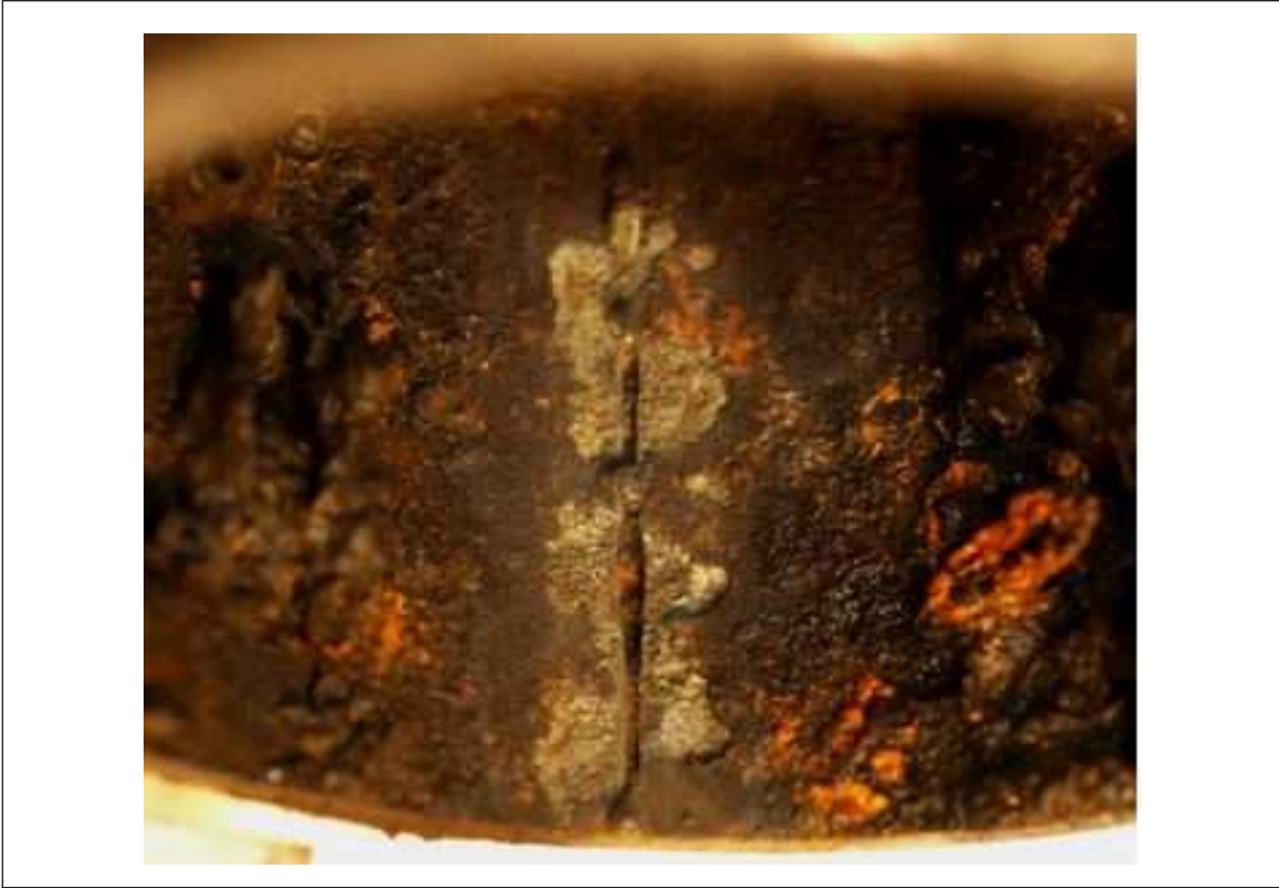
Fig. 11b. Leakage on an NPS 2½ steel sprinkler pipe in a wet pipe system after removal of corrosion products; preferential attack surrounding the weld seam is severe
