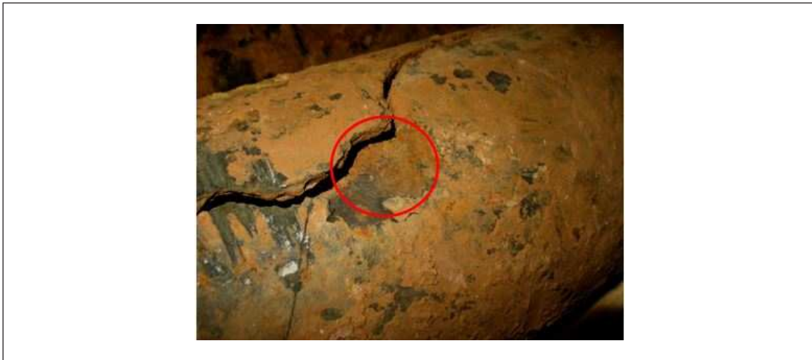
Fig. 7. Ruptured underground water main (identified as gray cast iron, 8 in. [20.3 cm] diameter) with cement lining on its inside diameter
