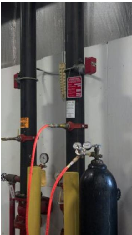
Pressurized cylinders provide nitrogen gas at sprinkler risers
