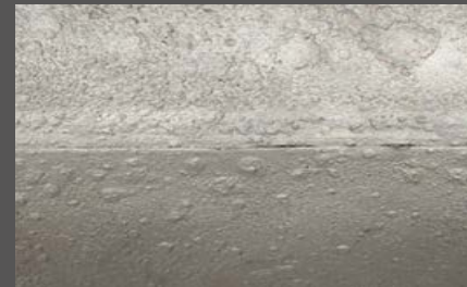
Corrosion on bottom of main
