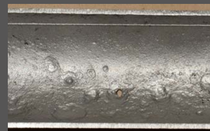
oxygen corrosion inside branch line
