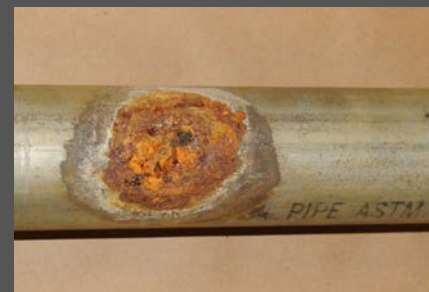
exterior of branch line leak
